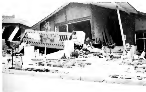
Photo 3. The upper portion of this split-level wood frame dwelling on Almetz Street has collapsed into the garage.
